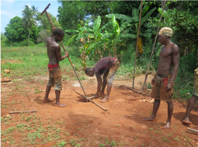
Workers in Makunduchi who are digging the hole (18 meters deep) to get fresh water for the well.
